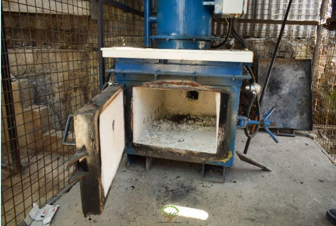
The Medical incinerator
